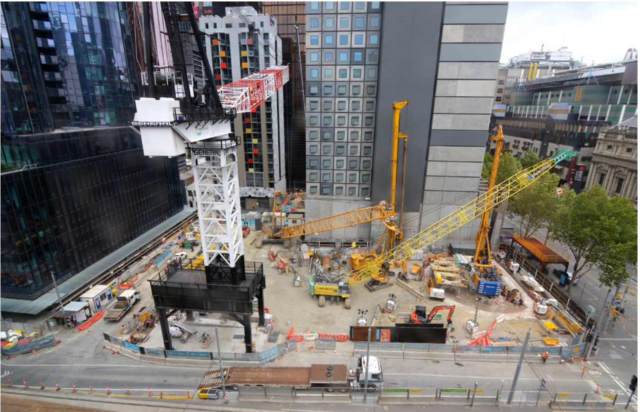
The tower crane recently installed at the La Trobe Street site (pictured left) will help facilitate construction of the future State Library Station.
